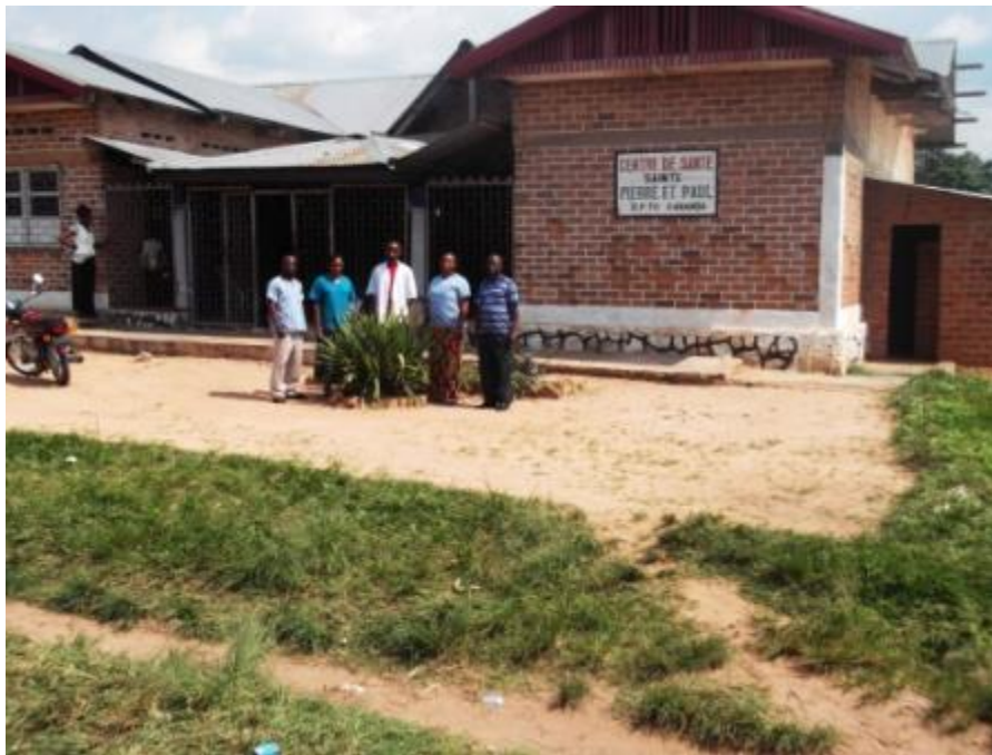
Annex to the building, showers and bathrooms for the nursing staff under construction
